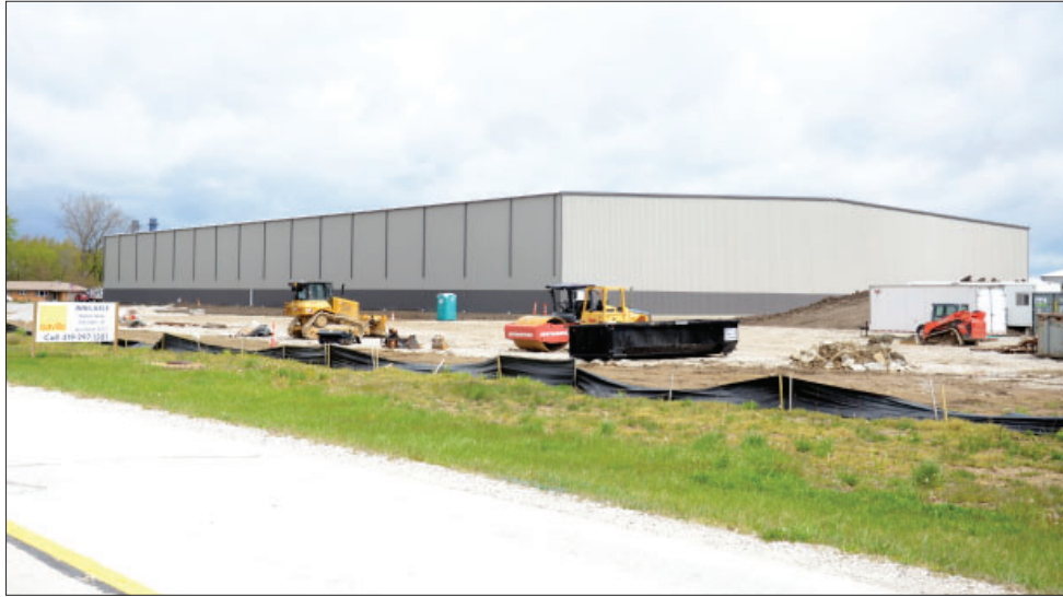
The 100,000-square-foot spec building is nearly completed. (Press photo by Ken Grosjean)
